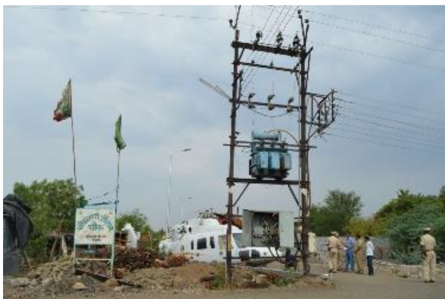
Fig:19 – 11 KV Electricity Transmission line
