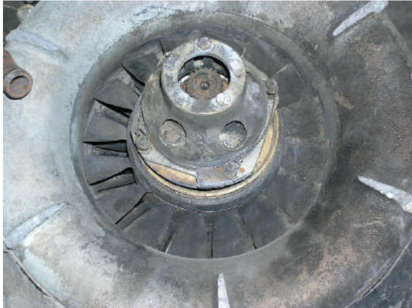
Compressor 1 st stage and No. 1 bearing housing, in-situ.
