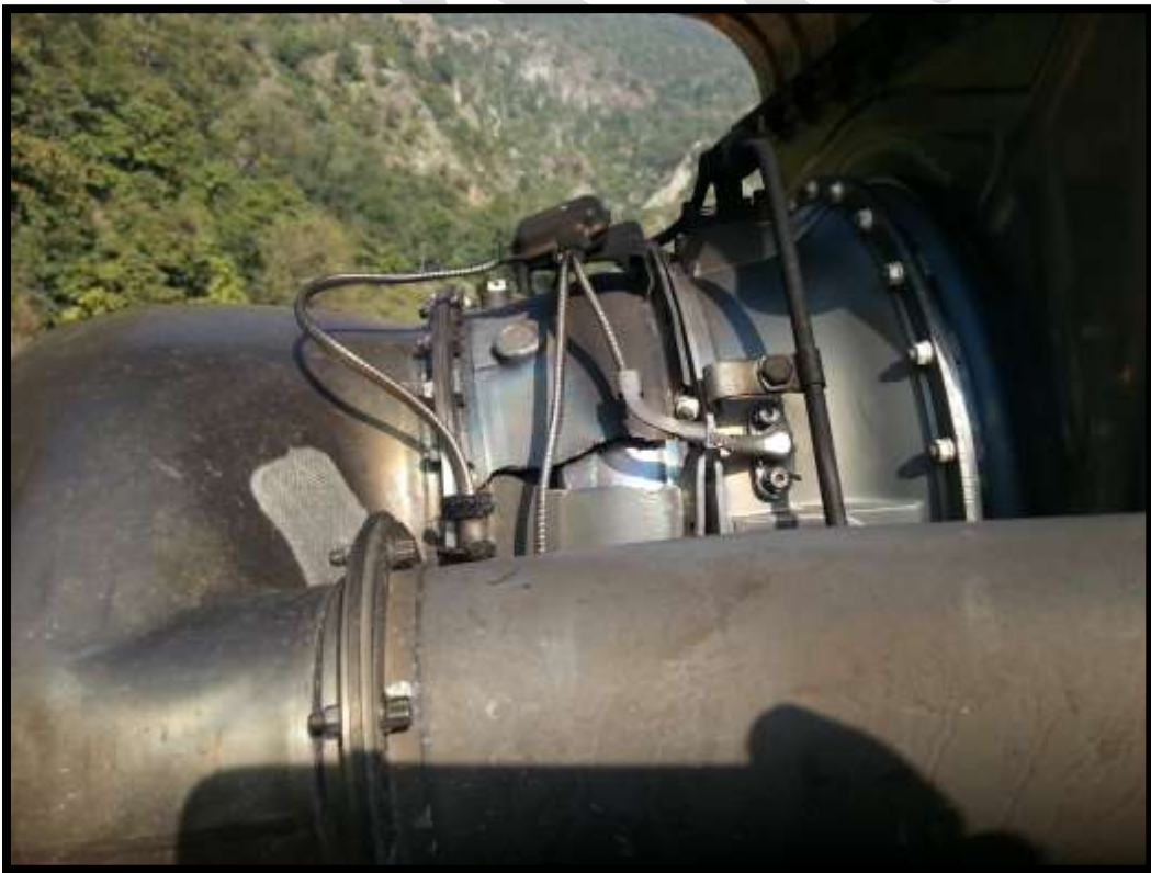
Damage to Engine
