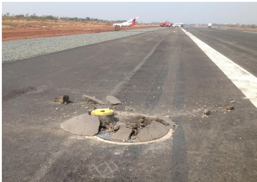
LH Gear Point of Impact with the runway lights
