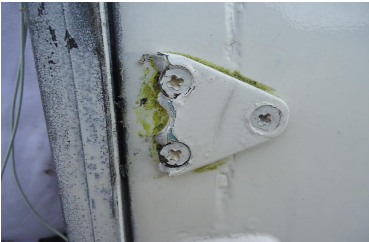
3. Flap door locking plates(upper & lower) were sheared off.
