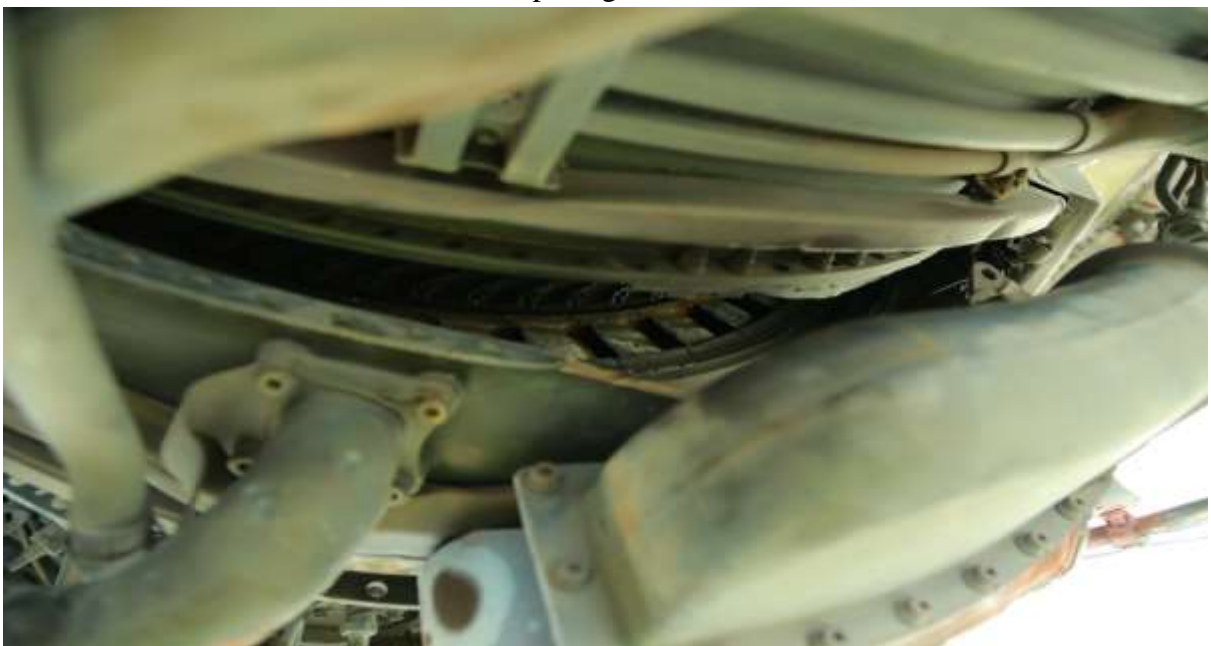
The High Pressure Turbine case breached
