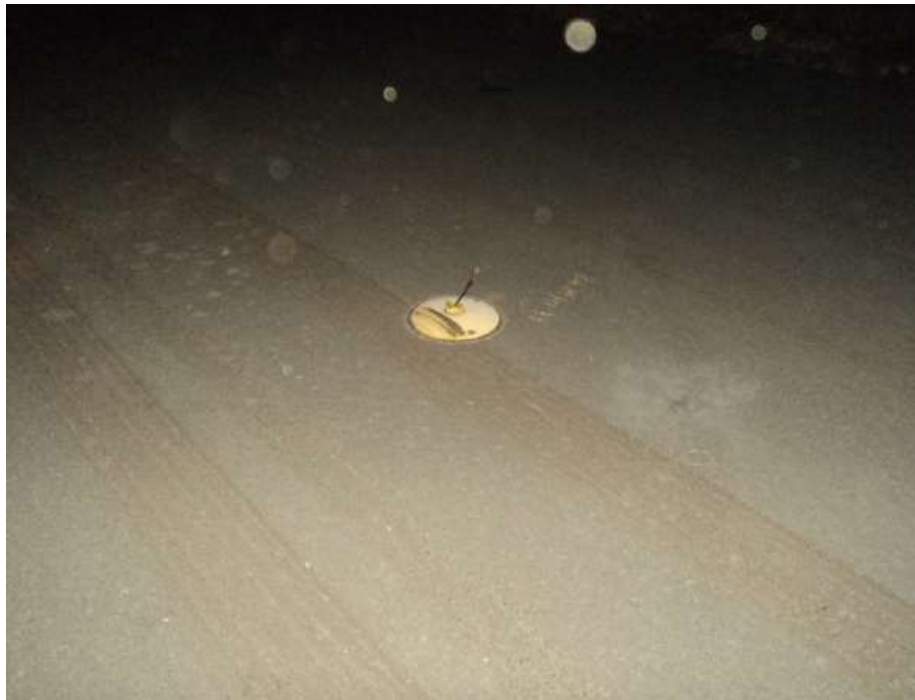
One of the damaged runway edge light
