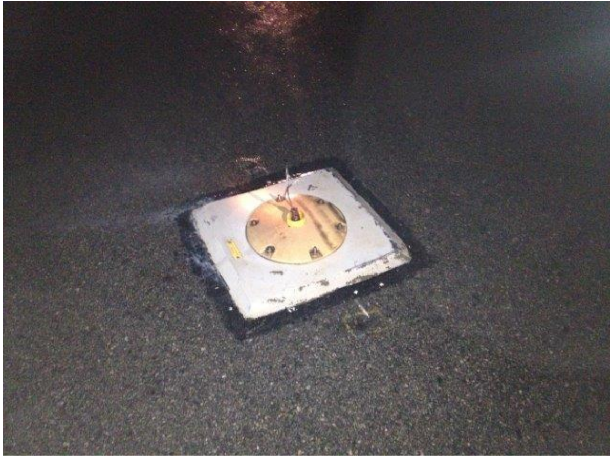
Damaged Runway shoulder edge light
