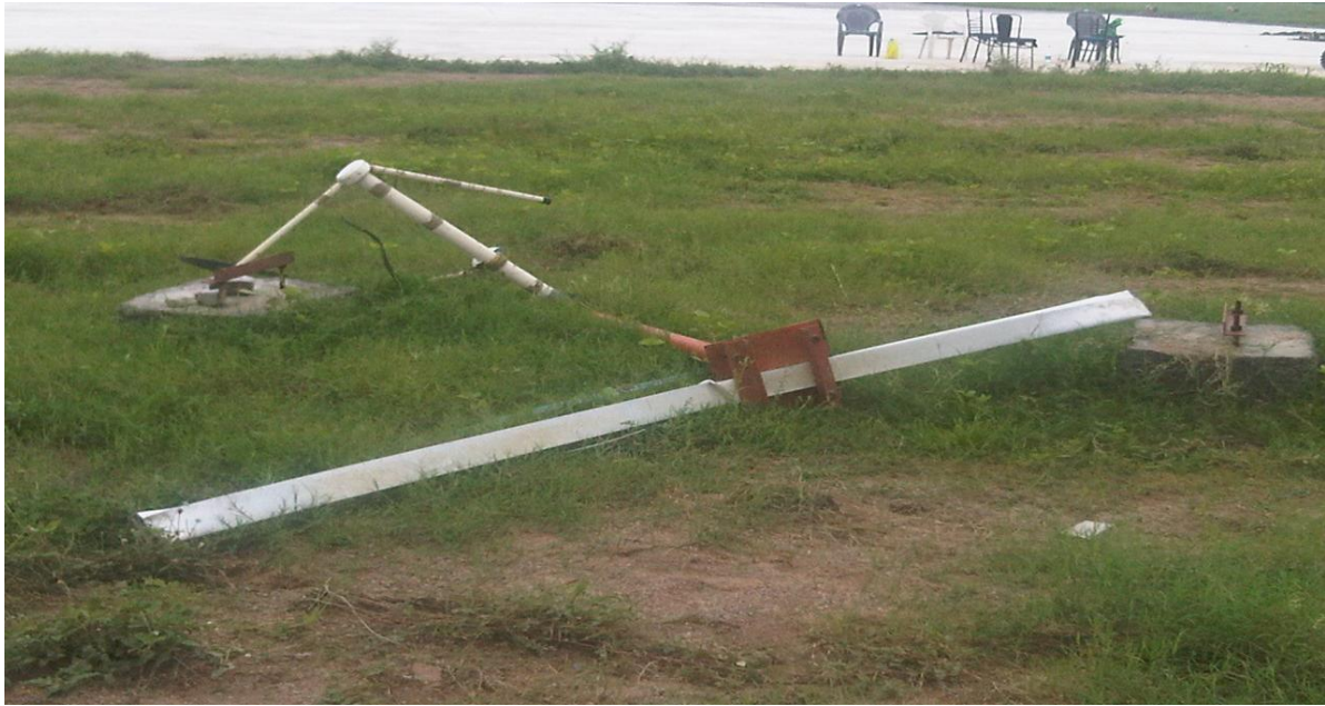
Figure: Damaged Localizer Antenna
